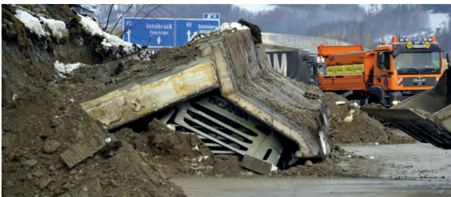
▲ Figure 1: The support structure on the day of the tragic collapse. (Image courtesy: Gabl and Pilch, 2015)
