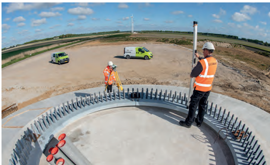
▲ Figure 4: An impression of surveying activities during the construction of a wind farm which today produces enough green electricity to supply 370,000 households. (Image courtesy: Geomaat)
